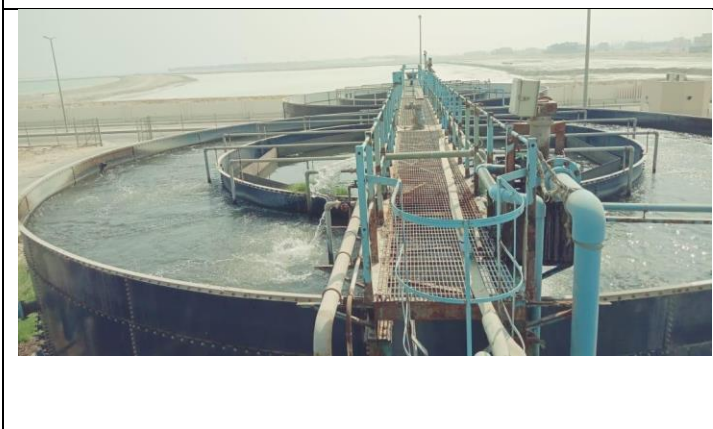
On campus biological water treatment plant at IAU
