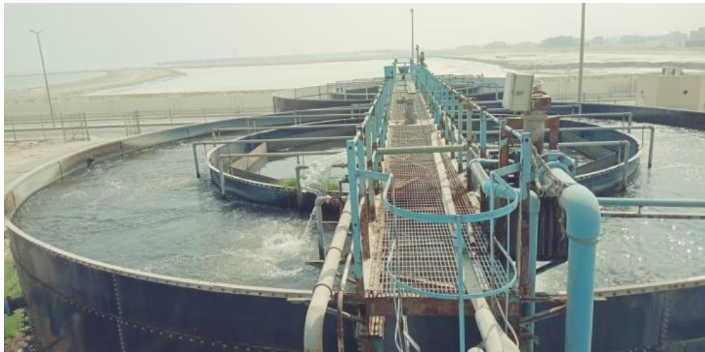
On campus biological water treatment plant at IAU
