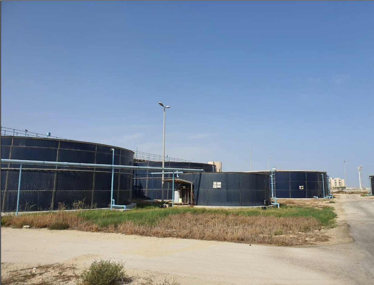
Recycled water processed in the tanks to protect ground water contamination
