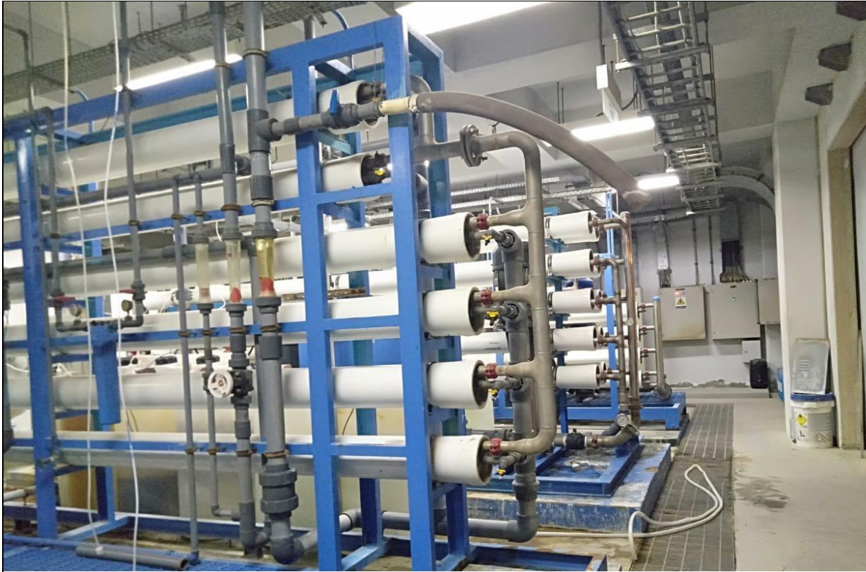
Water Desalination plant at IAU
