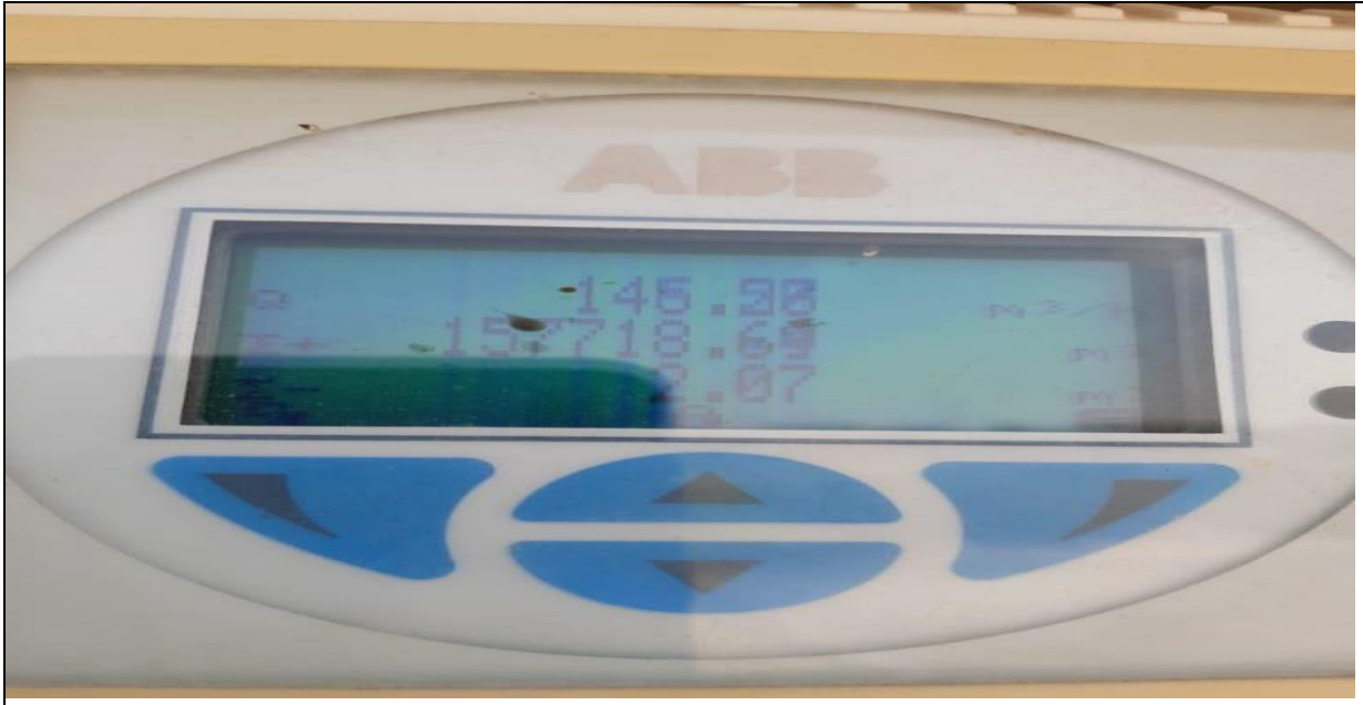
Water meter to regularly check water quality
