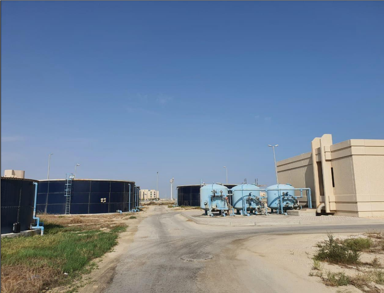
Water Pollution control system at IAU
