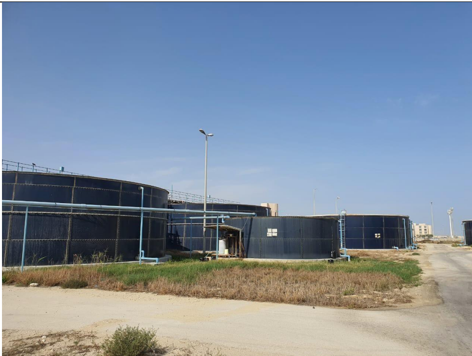
Recycled water processed in the tanks to protect ground water contamination
