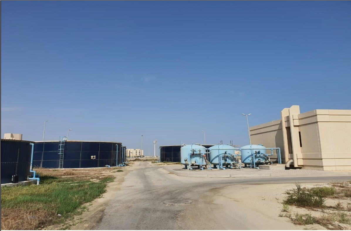
Water Pollution control system at IAU
