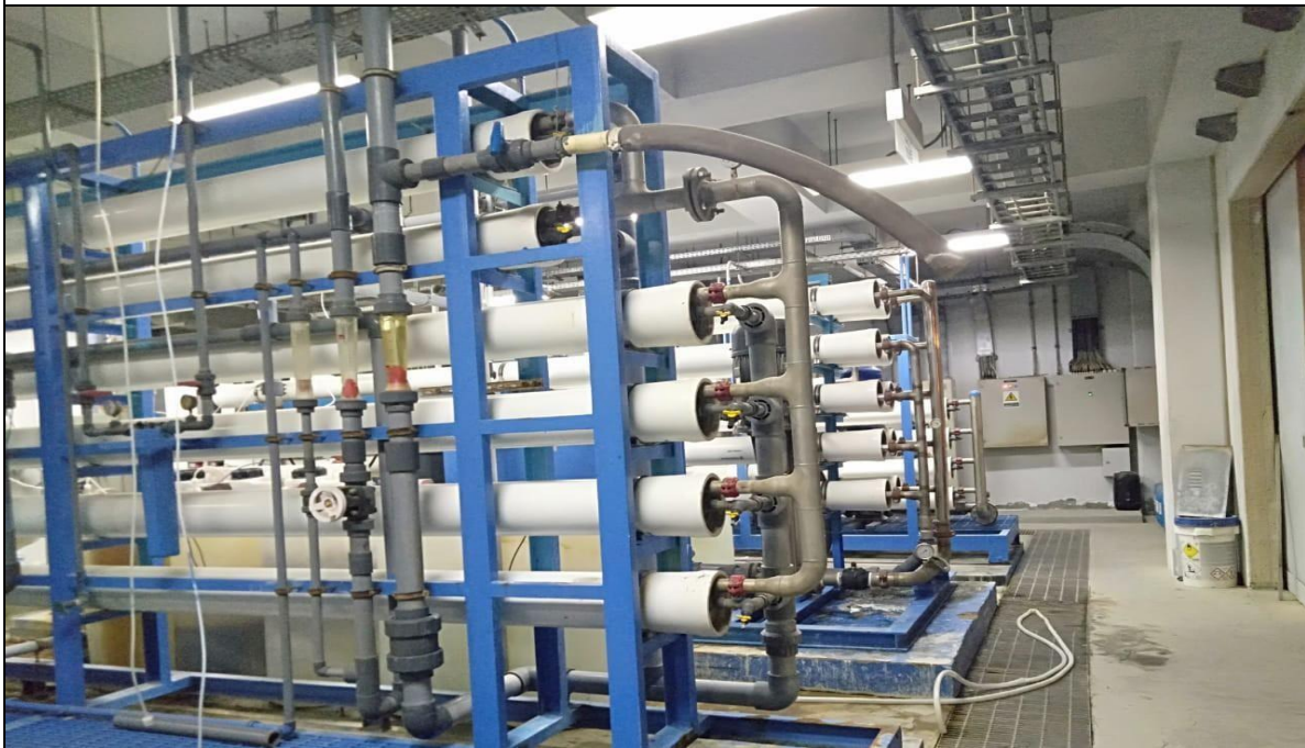
Water Desalination plant at IAU
