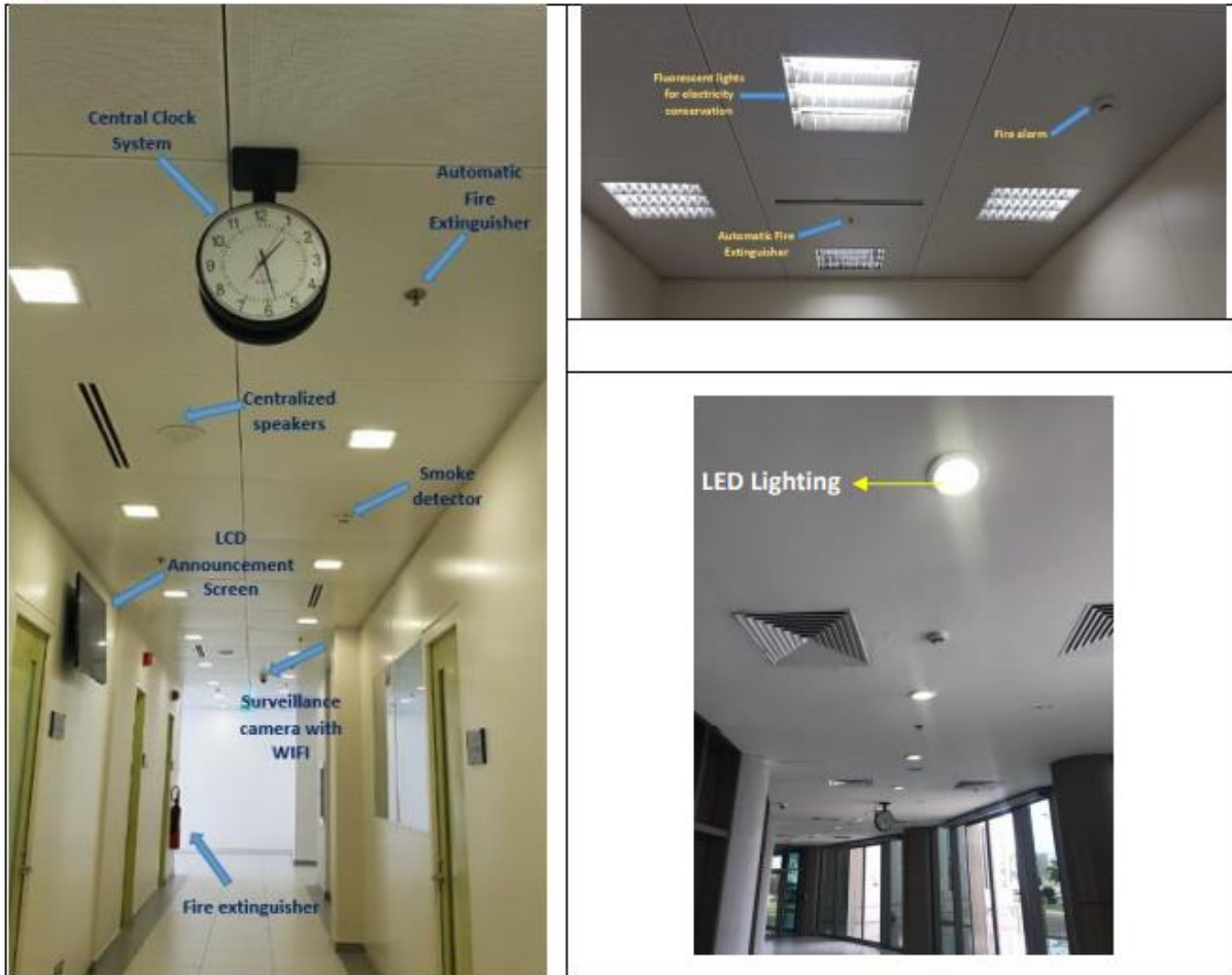
Energy Efficient Appliances Usage in all the Buildings of IAU: Use of LED & fluoracent lighting and lamps with central clock system, centralized speaker & LCD Announcement screen
