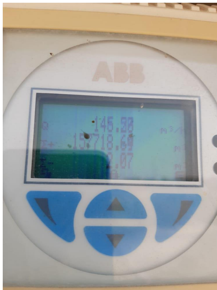
Water Meter to measure the water consumption in IAU
